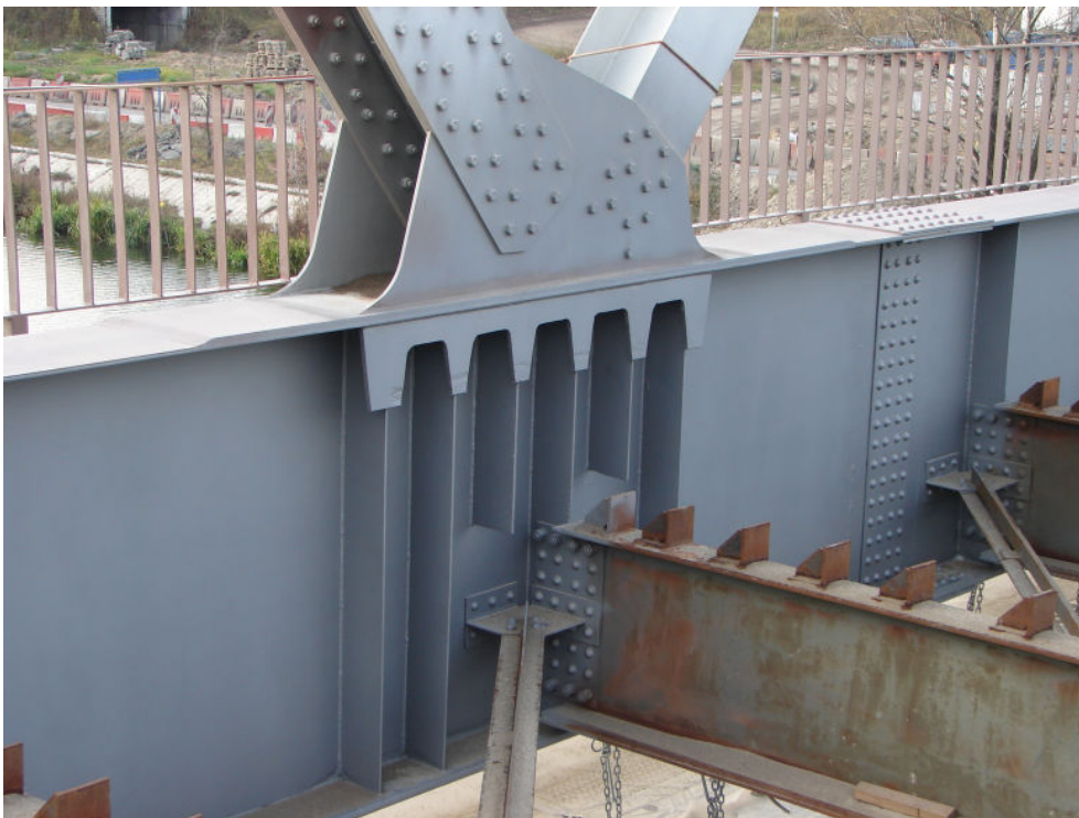
Fig.1. Bridge truss girder bottom flange – to – deck transverse beam and wind bracing structural connection
