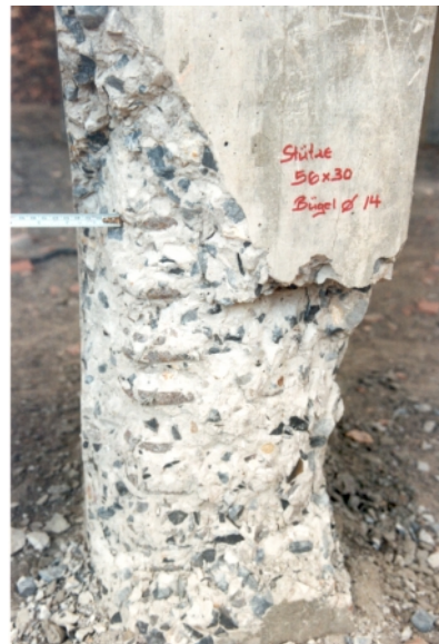
Damaged column base of ground floor
