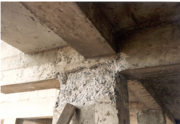
Damaged column-beam connection of ground floor
