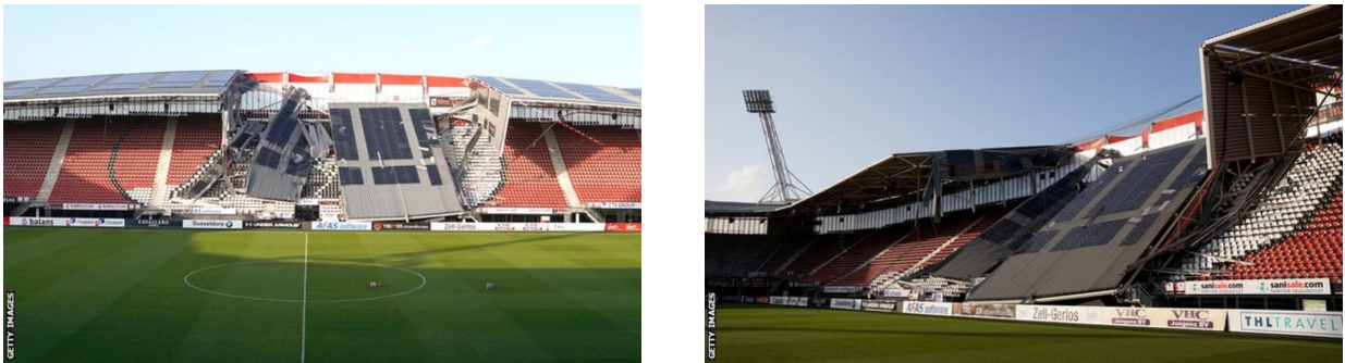
Figure 5.55: The collapse of AFAS football stadium in Alkmaar, Netherlands due to strong wind (Picture courtesy: BBC sports, 10 th August, 2019).
