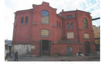
Andrey Vorontsov. "From the Historic warehouse of scenery for the Alexandrinka, two walls are remained - The News of Construction of St. Petersburg - Kanoner," Kanoner, September 19, 2010. Photo. Available from: http://kanoner.com/2010/09/19/17660/ (accessed February 13, 2017). Copyright: Kanoner, Andrey Vorontsov. The use of image is granted by the owners.
