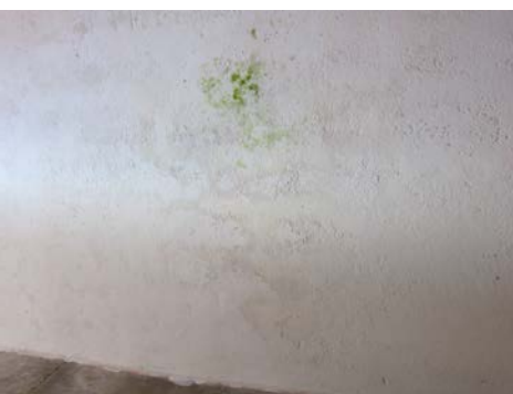
Infiltration on the wall. Author's file, 2013.
