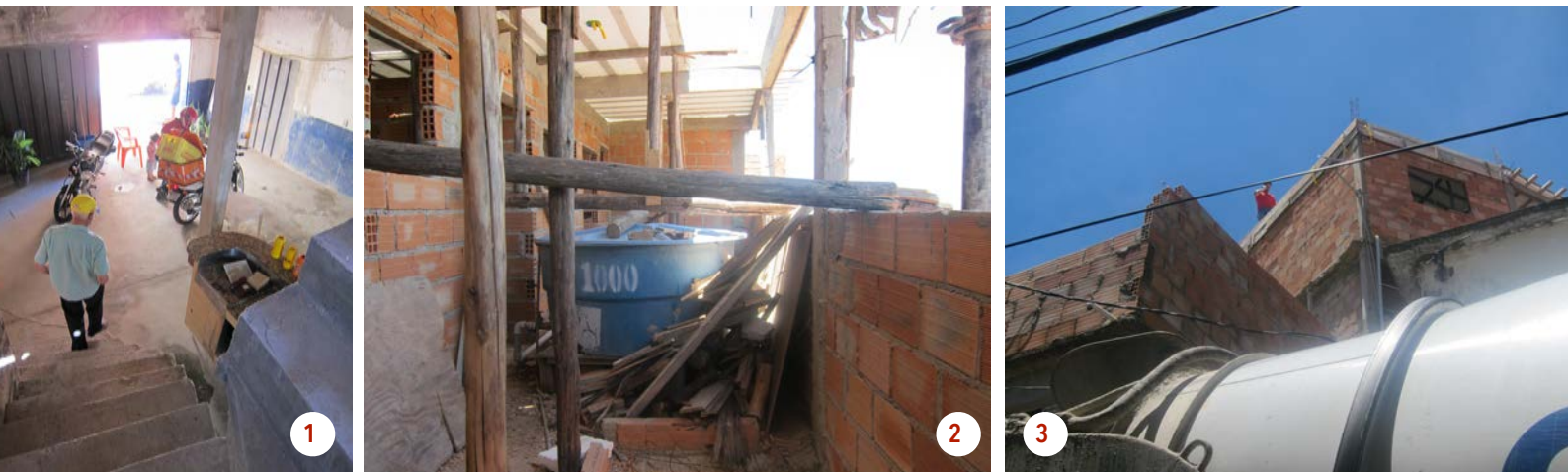
Insecurity in building sites. 1- Cintia's bar, stairs without handrails. 2-Levy's building site. 3-Levy's enterprise, Third slab, without parapets. Author's file, 2013.
