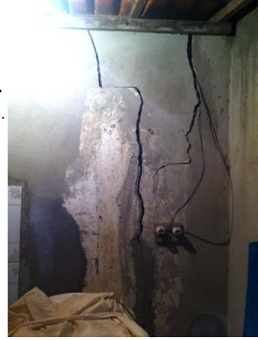
Crack in the laundry of Flavia's dwelling. Author's file, 2013.
