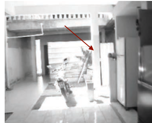
Eduardo's ground floor. The red arrow indicates the undesired column. Author's file, 2013.
