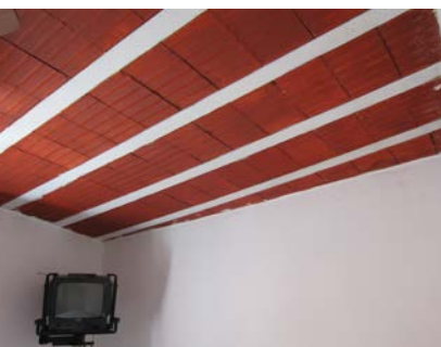
Precast slab, using reinforced concrete beams and ceramic bricks as infill. Author's file, 2013.
