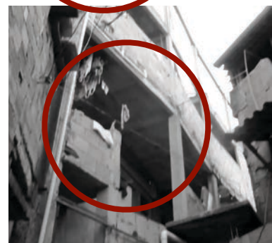
Absence of protection grill along stairs. Author’s file 2013.
