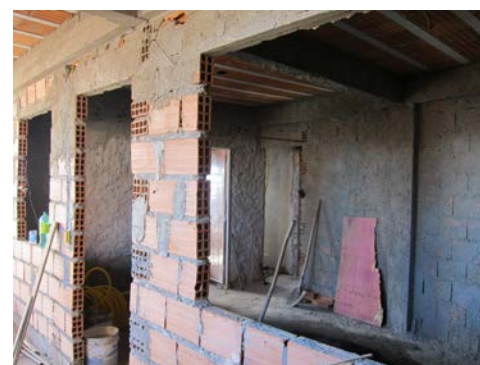
Windows and doors without lintels and sills. Author's file, 2013.
