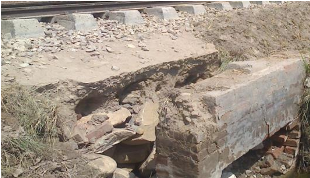
Figure 4-38: Embankment failure on the top of flood opening (over flow of water in culvert)
