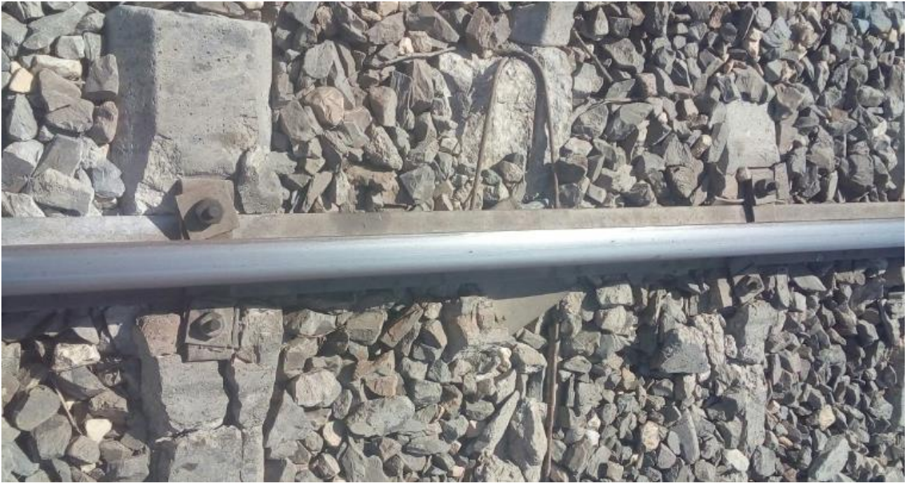
Figure 3-5: Crushed sleepers due to the fouled ballast
