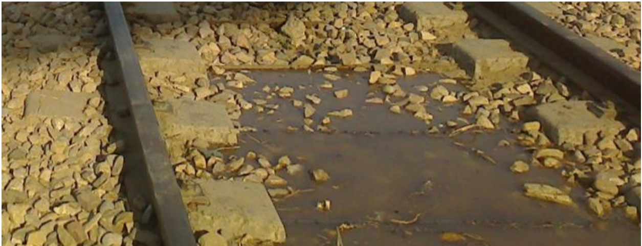
Figure 6-1: Rain water in the middle of track due to the poor drainage
