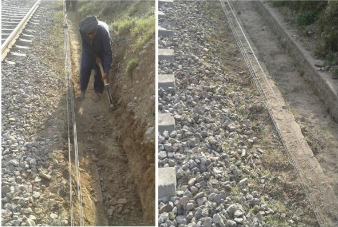
Figure 6-7: Inadequate side drains along the track (Rawalpindi-Lahore section)
