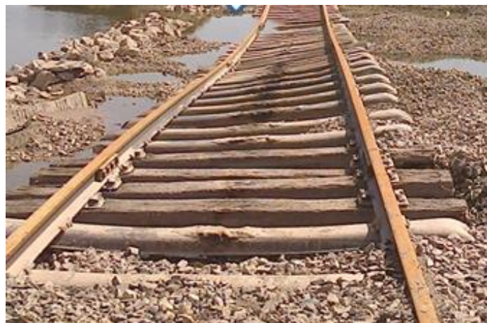
Figure 6-3: Track settlement due to the poor drainage
