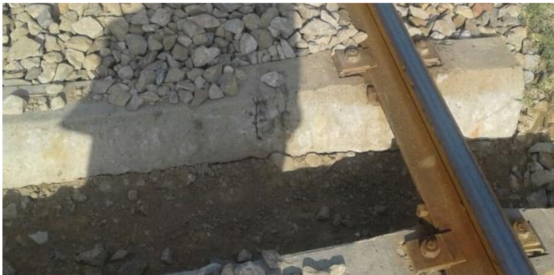
Figure 6-5: Cracked sleeper due to the underneath rigid surface (Fouled ballast)
