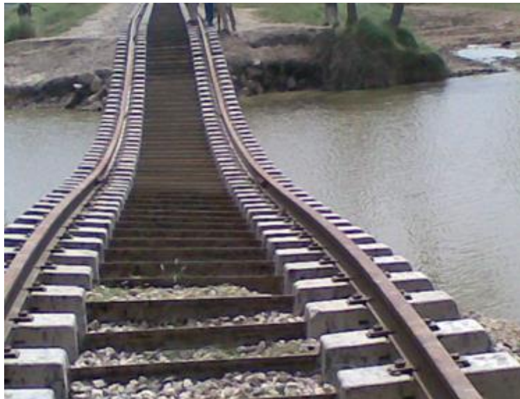
Figure 6-6: The formation washed away by flood water (Multan Division)
