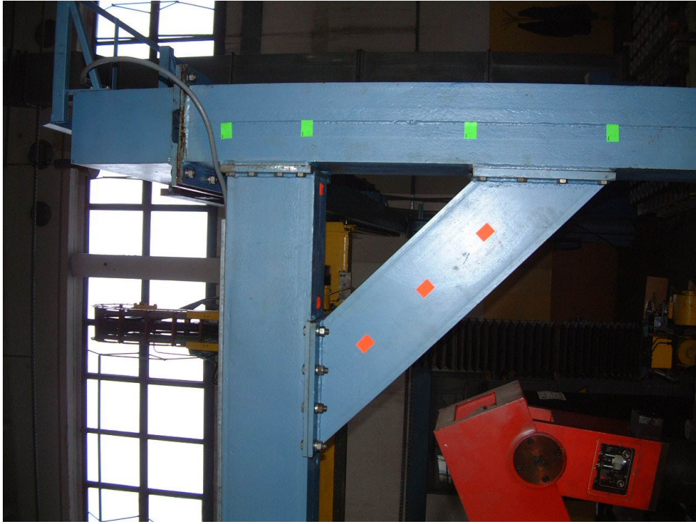
Figure 2: Location of damage, i.e. loosend bolts that connect the crosswise stiffening beam with the horizontal beam
