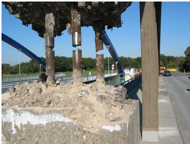
Figure 3: system modification: hanger cut through
