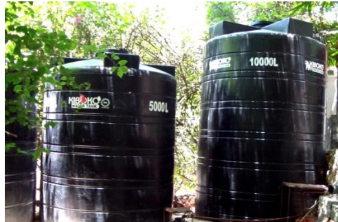
Figure 71: 5000 and 10,000 litre simtanks for storing water
