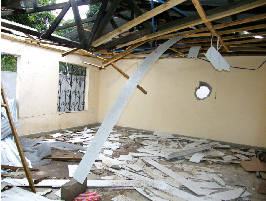
Figure 125: A house destroyed by accident bombes in Gongolamboto Source: Jafar Salehe ( Gongo-la-mboto reconstruction team project coordinator see Appendix 17 and 18)
