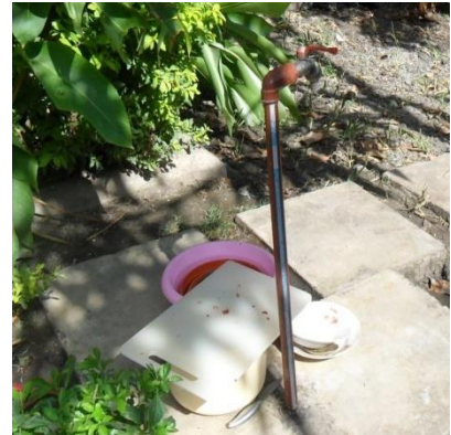
Figure 68: An outdoor water tap
